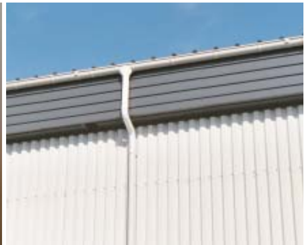
Rainwater is captured through these gutters and fed below ground into one of three 5,000 gallon tanks.
