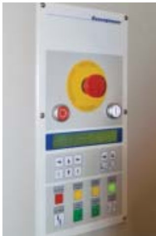
Controls for the washing system
