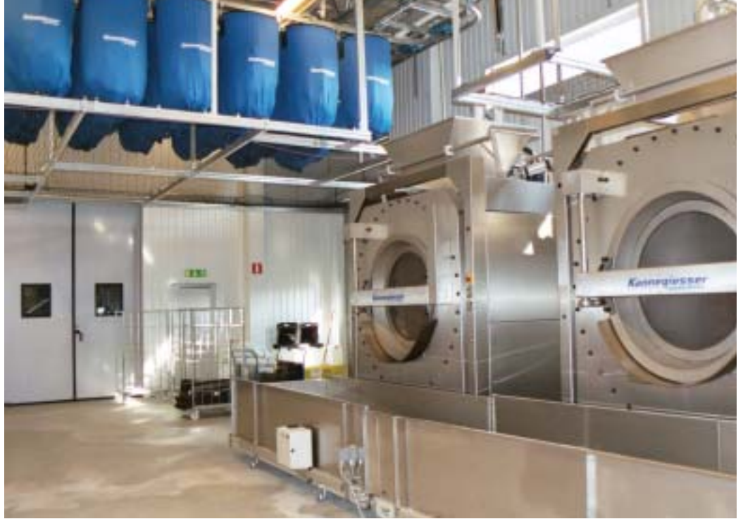
The washer/extractors have the capacity to wash 400 lbs. of mats. Mats are then dumped onto a conveyor system.
